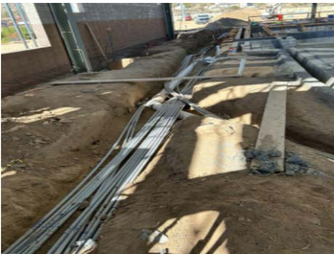
Pool Equipment Conduit to Main Electrical Room
